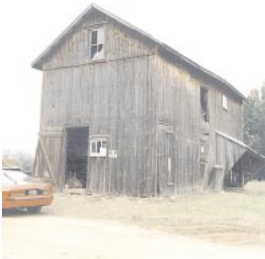
The wagon house, located on the east side of the main house off Upper Holland Road. Kathi did not inspect this structure closely but noted in the report that it appeared to be in good shape.
