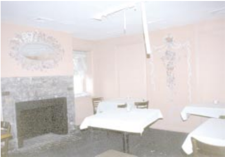
“Pink room”, located on the second floor of the main building. Fireplace mantel has been carefully removed, revealing the stone support system. Residents recall beautiful punch and gouge mantels on the fireplaces when the Spread was still open for business.
