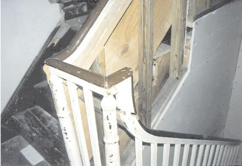
Details of the original Federal balusters, newels, and railing located in the rear of the building between the second and third floors. Kathi noted that only finer homes of the period had staircases of such elegance.
