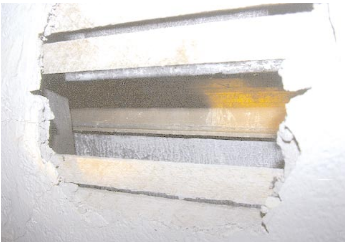
Kathi Auerbach discovered the original Federal chairrail behind a false wall in the rear stairwell. (Right) In this photo Kathi noticed two different kinds of lath; hand-split and circular sawn, indicating a later patching when
