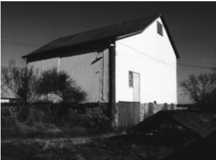
A Northeast view of the barn. The barn is in excellent condition.
